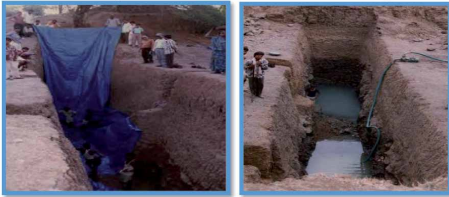
Figure 9. Artificial groundwater recharge structure at Rajgarh district in MP.
