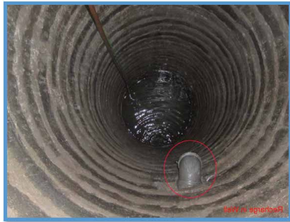
Figure 4. Dug well groundwater recharge structure.
