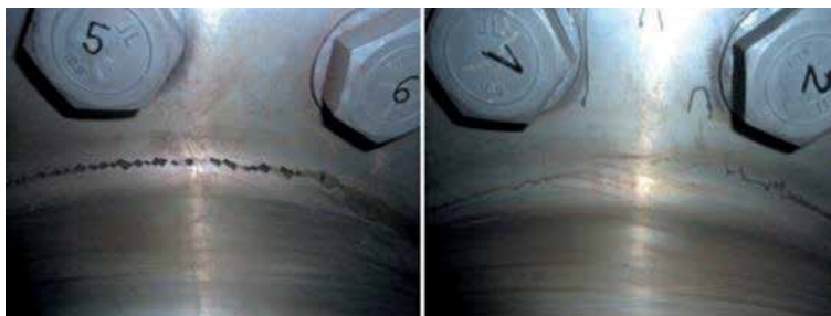
Figure 2. Fracture of hoist's shaft [8].
