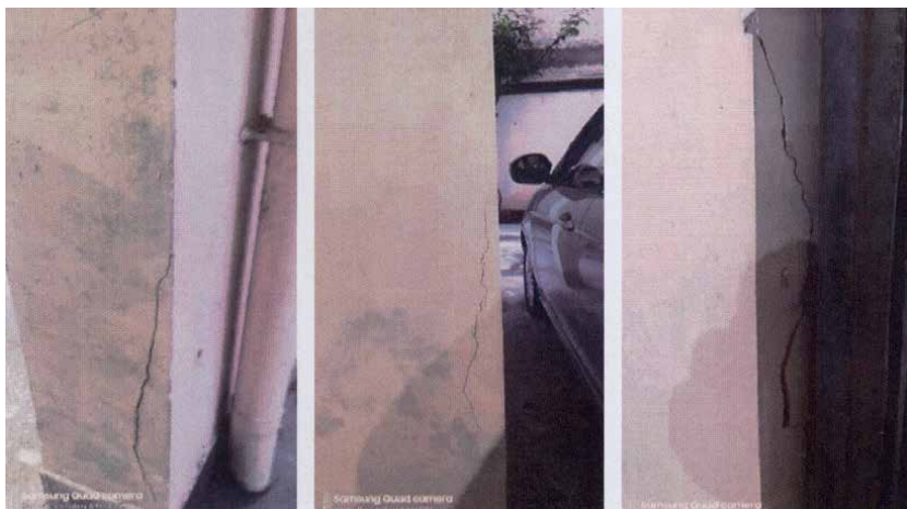
Figure 5. Typical distress in ground level columns caused by rust in ribbed TMT bars in a 10 year old building in Kolkata.
