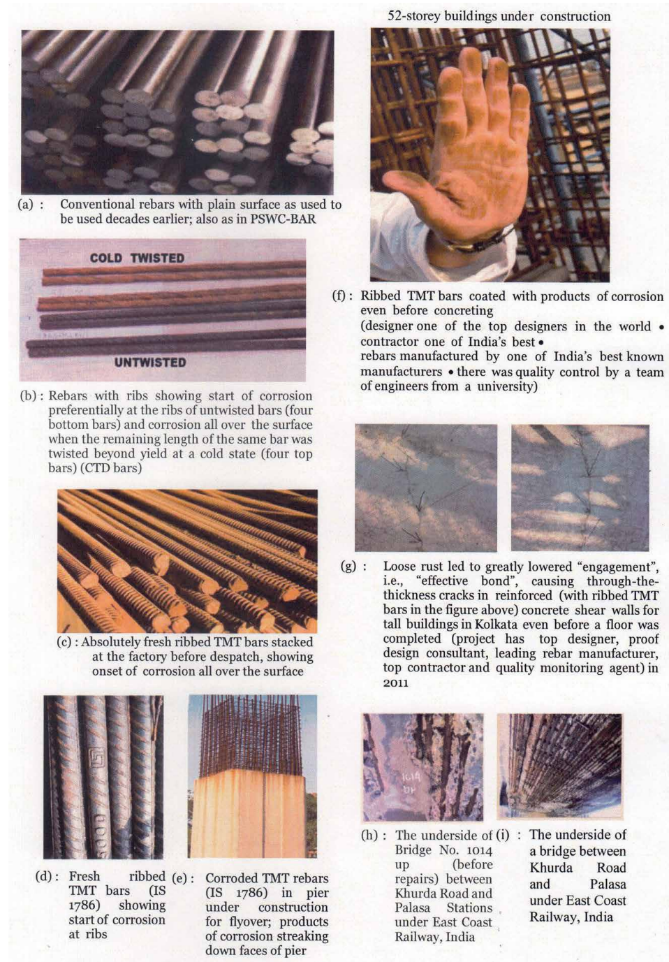
Figure 6. A collection of plain bars free from rust and ribbed CTD and TMT bars with various stages of corrosion.
