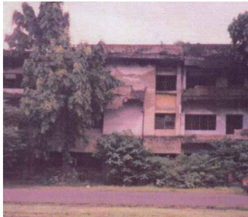
Figure 4. Abandoned hospital building a decade after construction in the new township of Salt Lake City, Kolkata.
