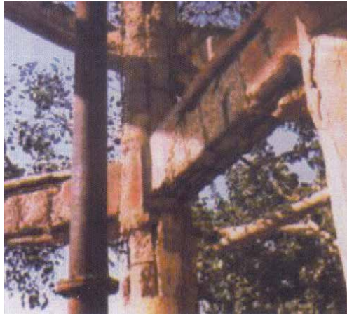
Figure 3. Distress in staging of overhead water reservoir due to corrosion in rebars.
