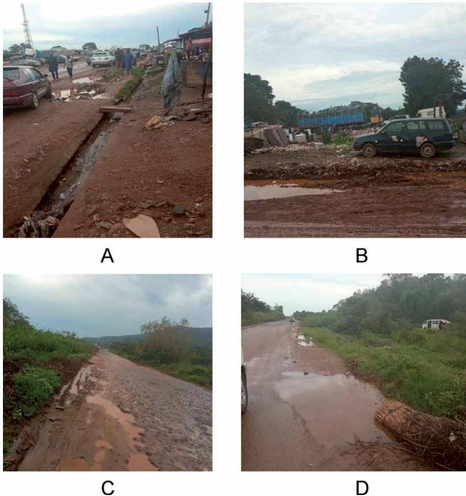
Figure 3. A section of Enugu – Port-Harcourt Express Road, Lokpanta, Imo State. This section of the road reveal typical South Eastern Nigerian road that is supposed to be maintained by the Federal Government headed by President Mohammed Buhari. The failure of government to be functional created the observed collection of water, blocked drain, mud, solid wastes, grass, stuck vehicles, used tyres and squalid environment all of which provide perfect environment for mosquito breeding and optimized malaria transmission (A–D).
