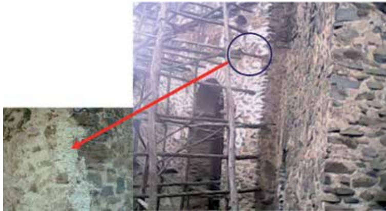
Figure 5. Mortar repointing used during the restoration of the palace [source; Eskinder Desta].
