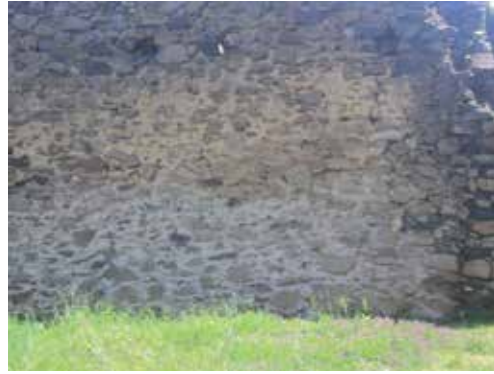
Figure 4. A widespread lack of binding mortar in between the stone masonry [source; Eskinder Desta].
