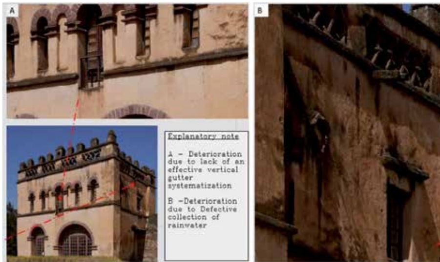
Figure 2. The effect of improper rainwater removal on the face of the wall [29].
