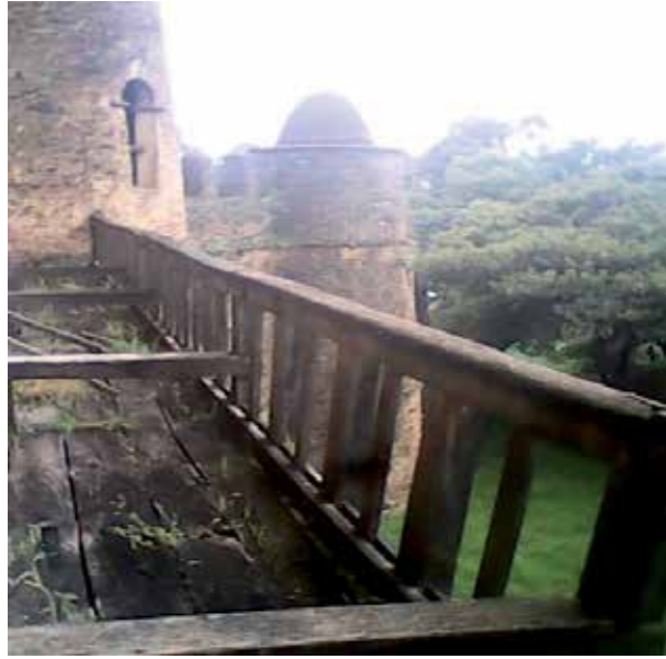
Figure 6. Active durability issue due to the presence of grass and alga on the wood floor terrace [source; Eskinder Desta].
