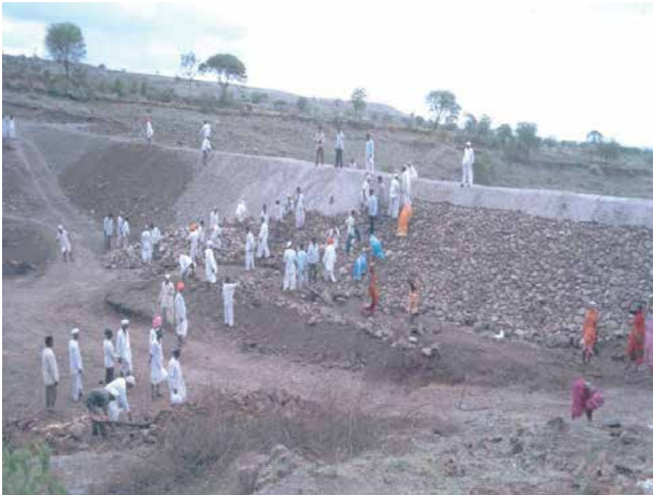
Fig. 5. Stone Pitching on the face of the earthen bund of a percolation tank under construction. Photo from village Hivre Bazar, District: Nagar, Maharashtra state.
