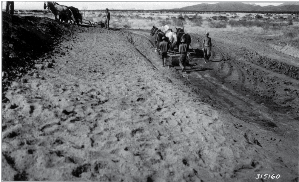
Fig. 4. Construction of stock water storage tanks at the Jornada Experimental Range using three-horse Fresno teams on Big Meadows tank by the Civilian Conservation Corps (CCC) in April 1934.
