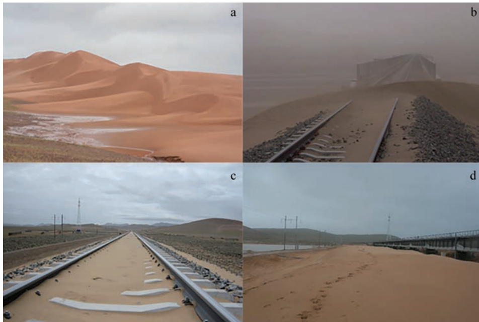
Figure 1. Sand disasters along the Qinghai-Tibet Railway. (a) Hongliang River section, (b) Tuotuo River section, (c) Za'gya Zangbo section, (d) Cuona Lake section.
