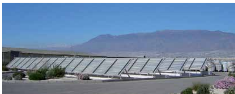
Fig. 13. View of the solar detoxification demonstration plant erected by ALBAIDA at La Mojenera (Almería, Spain), (Malato et al., 2007).
