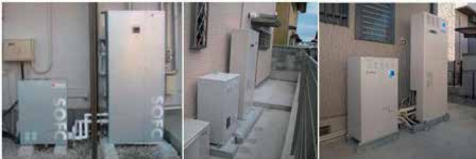
Fig. 7. Appearances of installation sites of residential SOFC CHP systems under demonstrative research project in Japan (Hosoi et al., 2011).
