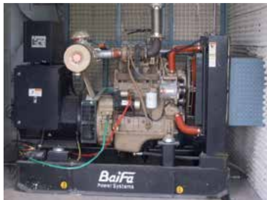
Fig. 16. Internal combustion engine-generator for power generation
