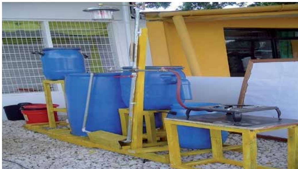
Fig. 4. A biogas plant using plastic containers (Source DIT R&PGS-2011)
