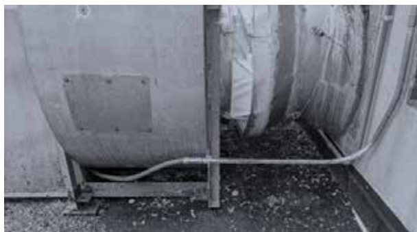
Figure 3. Pigeon nests under a HVAC machine on top of the Biology building on TTU campus.
