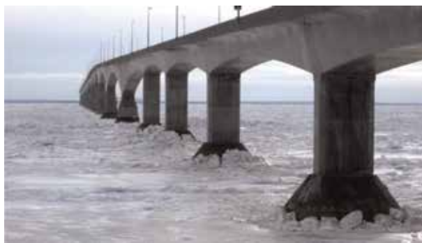
Figure 1. The ice cover around bridge piers (the confederation bridge, Prince Edward Island, 2015).
