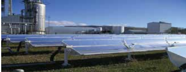
Fig. 23. ACUREX solar plant
