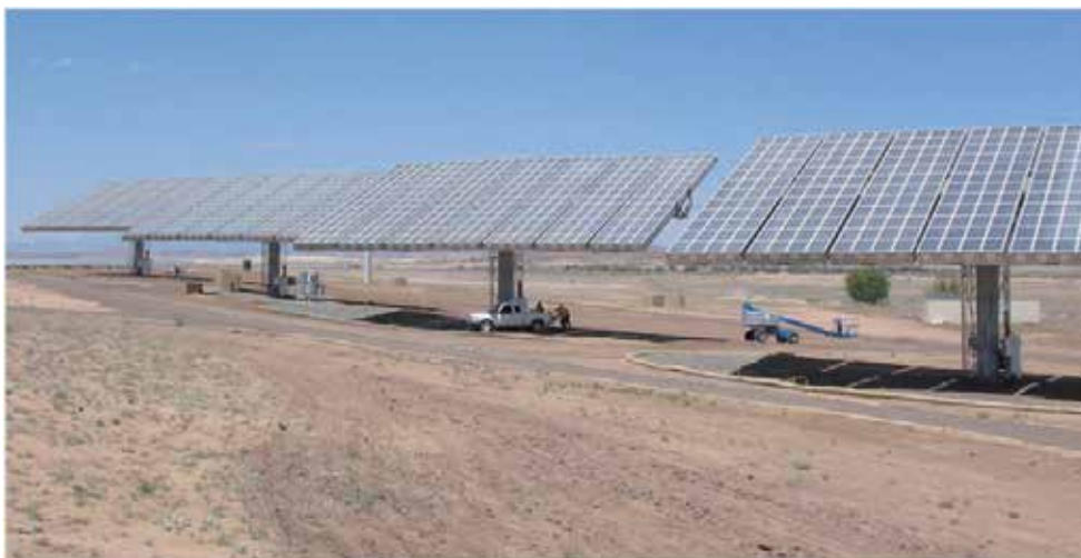
Fig. 2. Several 35-kW CPV systems built by Amonix in Torrance, California were installed at a Public Service power plant in Arizona. The system uses Fresnel lenses to concentrate sunlight onto high efficiency silicon solar cells. The pickup truck in the shade gives an idea of size of this installation.
