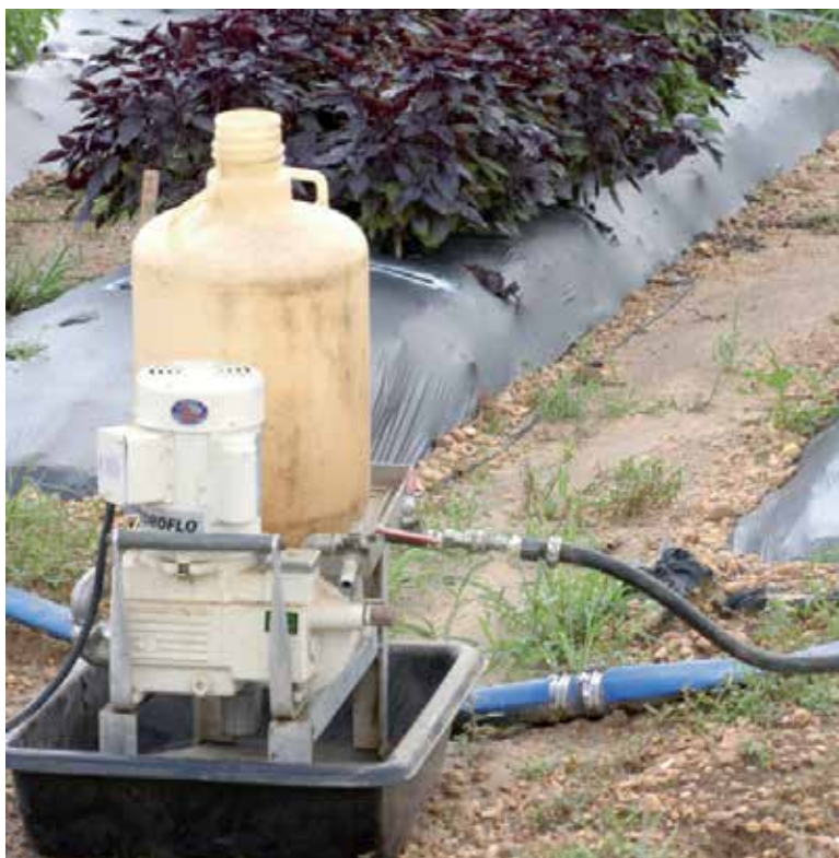
Fig. 7. A positive displacement electric (1/3 hp) metering pump with a 5-gallon jug for the concentrated insecticide solution and a containment tray beneath to catch all drips, spillage, etc. In the center of the picture is a flush valve to quickly and completely rinse all solution from within the pump.
