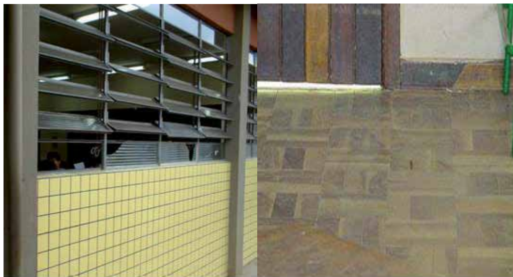
Fig. 18. Classroom com broken window panes and spaces between the door and the floor
