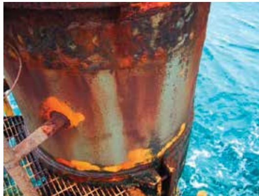
Figure 3. Degradation of offshore structural component [3].
