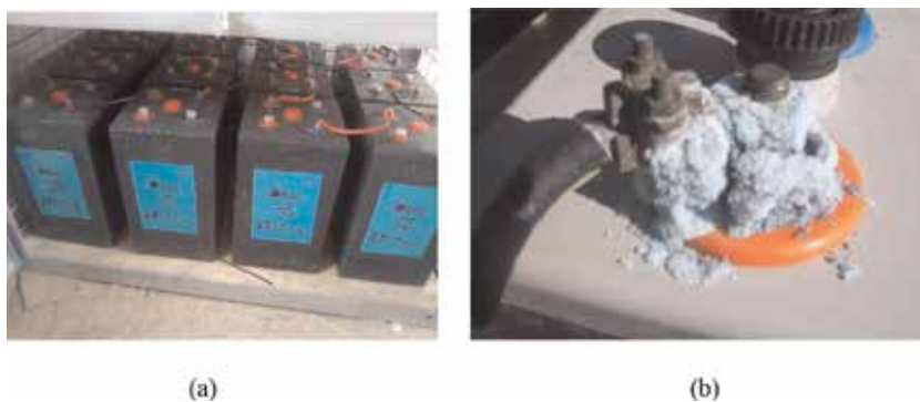
Figure 9. (a) Deep discharge of batteries and (b) sulfation of batteries due to lack of maintenance.
