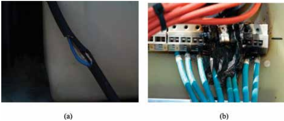
Figure 7. (a) Wiring system fault and (b) poor tightening of connections fault.
