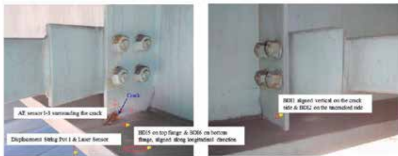
Figure 4. Crack locations and sensor placements: (a) details at G 3 B 2 D 3 and (b) details at G 3 B 3 D 3 .
