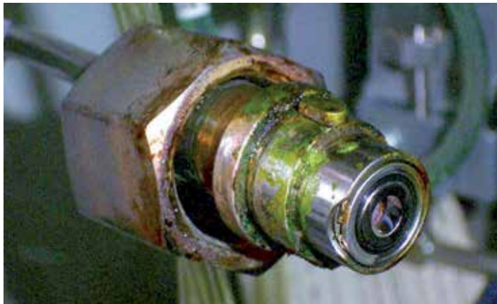
Fig. 6. Green hypochlorous and hydrochloric acids from chlorine corrosion.
