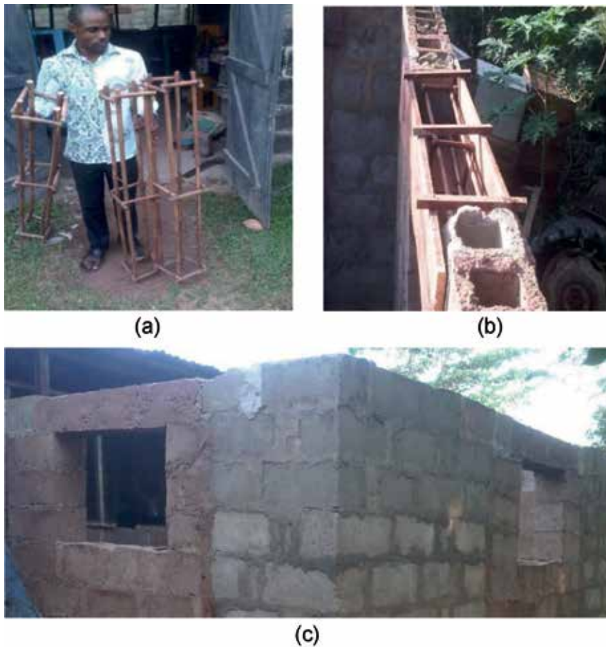
Figure 15. (a) Rattan cane reinforcement, (b) lintel beam casting in progress, (c) the cured concrete lintel beam after 28 days. Source: [23].
