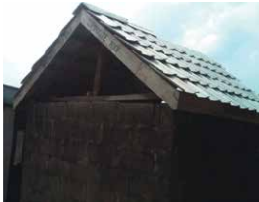
Figure 6. Fibre-reinforced composite roofing tiles installed on a gable-roofed building in Ibadan, Nigeria. Source: [23].
