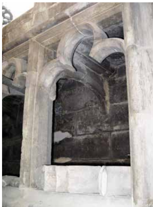
Figure 2. Repaired tracery with damaged elements in Notre Dame du Sablon (photo by M. Drdácý).
