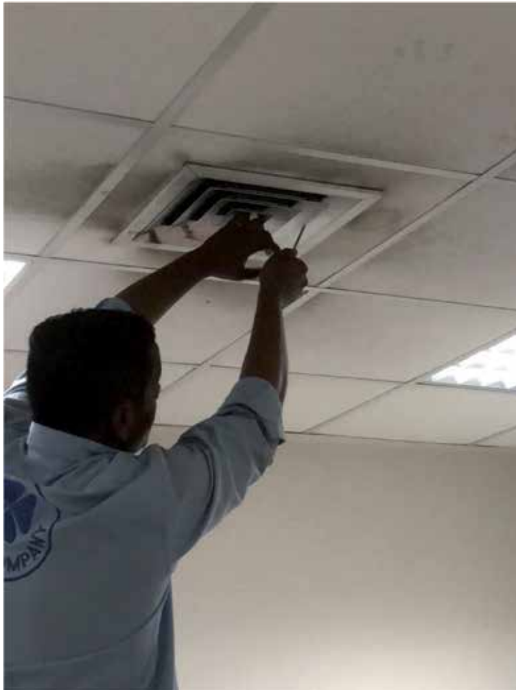
Figure 9. Ducts should be cleaned periodically.
