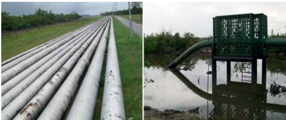
Figure 5. Crude oil pipeline and well head situated in reclaimed coastal area in the Niger Delta, Nigeria.
