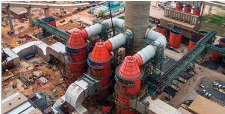
Figure 5. Eskom's Kusile wet flue gas desulphurisation plant (South Africa). Image: Biznis Africa (2018).
