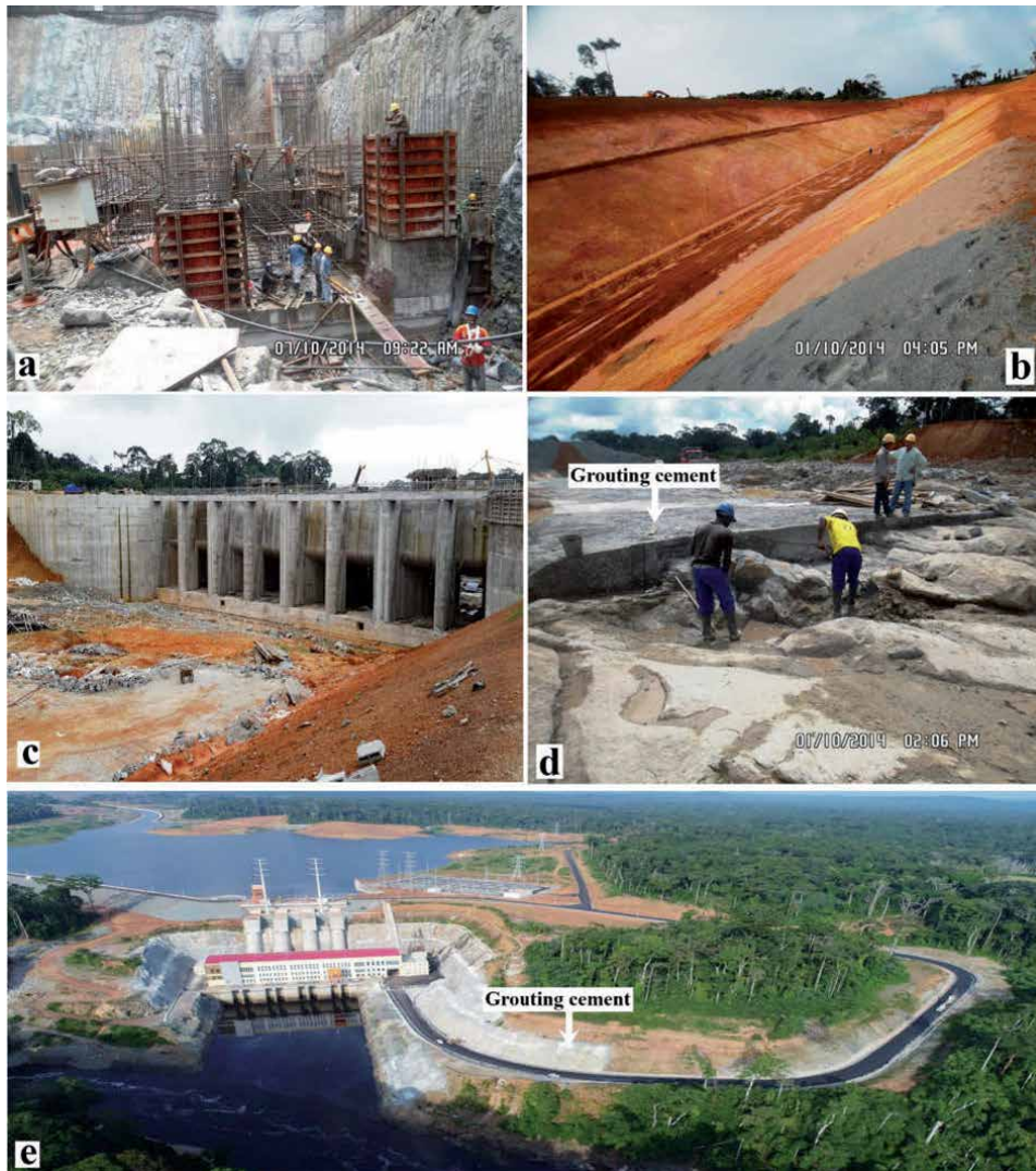
Figure 8. (a–c) Display different usages of Ntem formations and quaternary soil deposits; (d and e) amendment of Ntem formations and slope formed by quaternary soil deposits with grouting cement.
