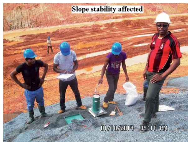
Figure 5. Slope stability affected by raining water.
