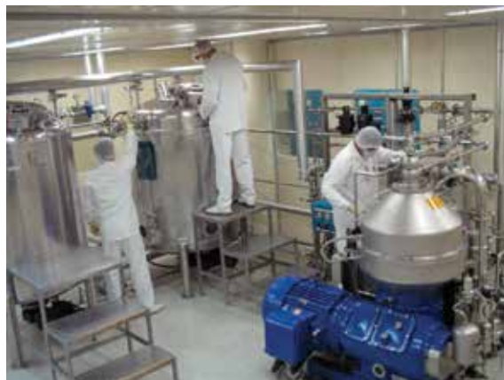
Figure 1. Partial view of plasma fractionation production plant of antivenoms and antitoxins (Instituto Butantan Foundation).
