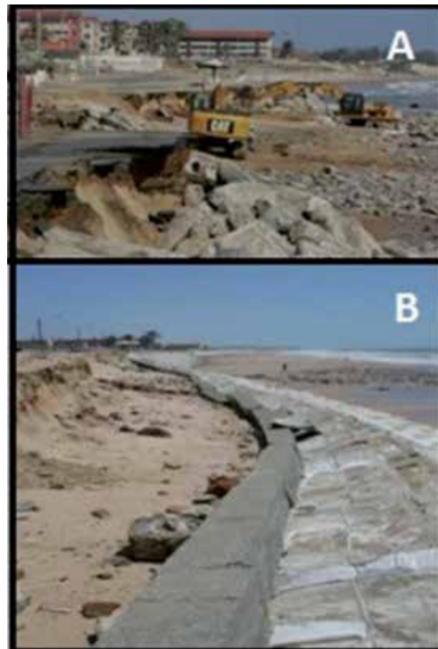
Figure 6. (A) Erosion in Icarai Beach, 25 km downdrift of Mucuripe harbor, resulting from the interventions in Fortaleza city and in the area around the harbor. The rising of the sea must also be a factor producing the erosion. (B) Bag-wall installed in Icarai Beach in the 2010s, already destroyed by the waves.
