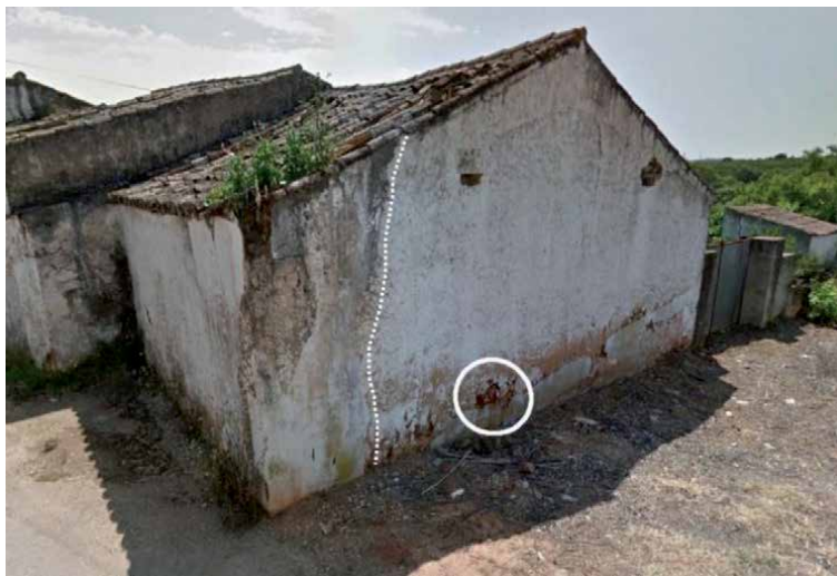
Figure 10. Fonte de Louzeiros, building of class A rebuilt after the 1969 earthquake, showing the repair mark of a corner failure (dotted line). Inside the white circle is visible the red color of the clay used to join the adobe masonry. Source: Google Earth.
