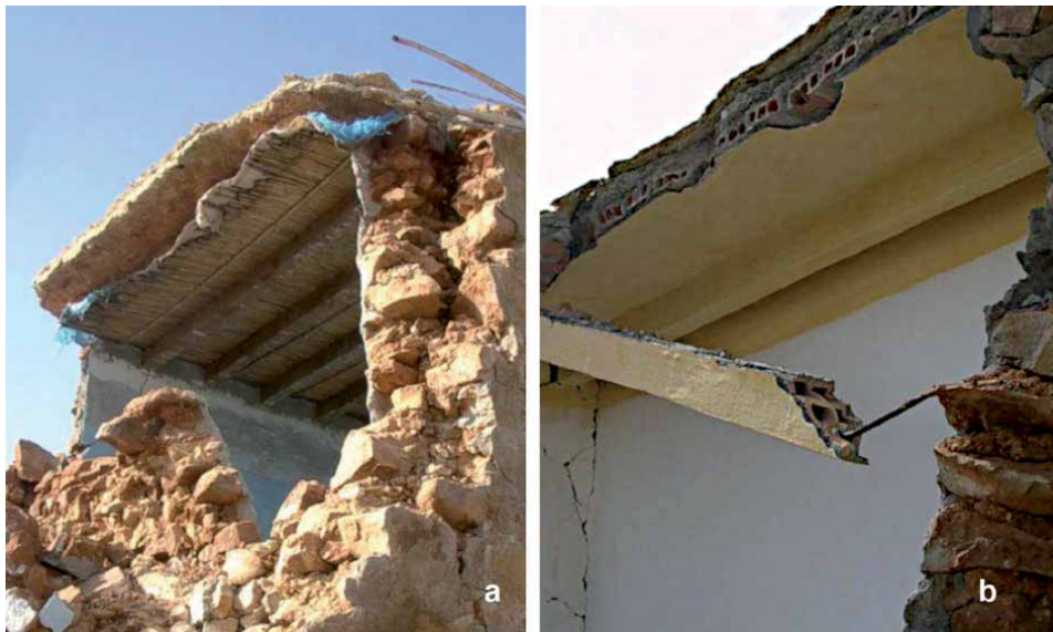
Figure 13. Ait Kamra, traditional house pattern: (a) partial collapse showing the double-leaf load-bearing walls, fieldstone masonry bonded with mud mortar and roof of wooden logs and canes covered with a plastic film (blue) and layer of water-repellent mortar (grade 4, class A); (b) handmade joist of hollow bricks assembled with a single steel rod. Source: P Murphy.
