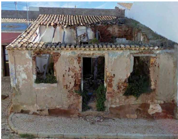
Figure 7. Vila do Bispo, typical house of vulnerability class A built with raw materials: load-bearing walls made with adobe bricks, doors and windows with lintels, and wooden logs supporting a tiled roof over a bed of reeds. Source: Google Earth.
