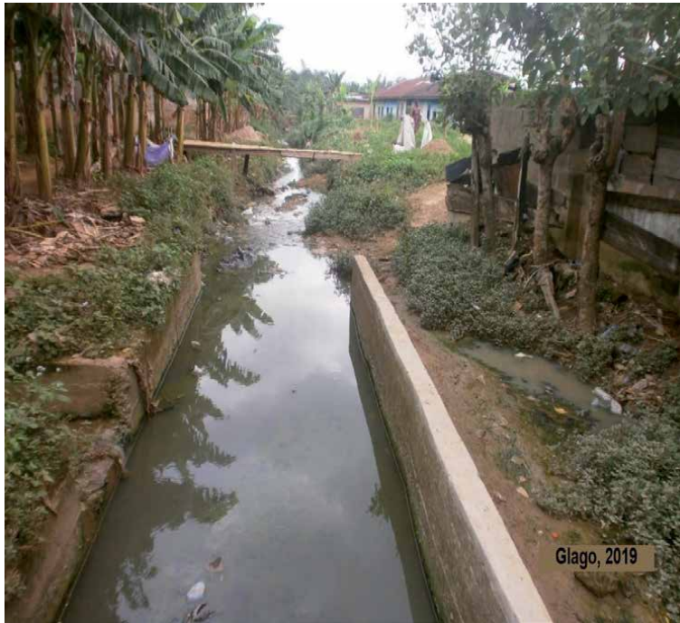
Figure 1. Showing a partially completed drain in the Asamankese community, Eastern region of Ghana. Source: Author.
