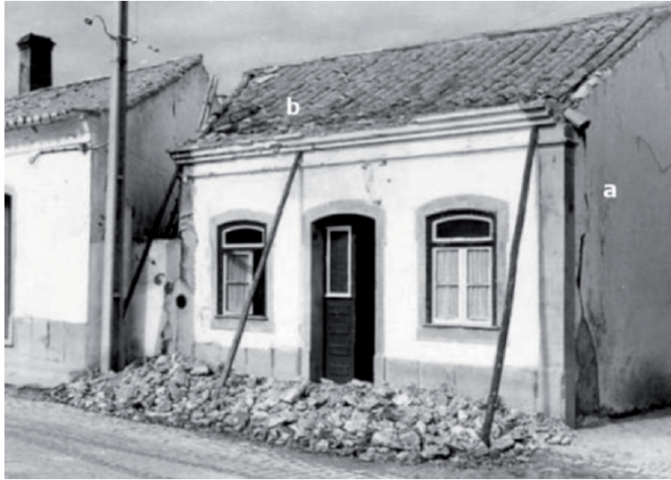
Figure 8. Sagres, building of class A with damage of grade 3: (a) loss of connection of load-bearing walls with drift of façade, and (b) detachment of cornices and tiles with partial roof collapse. Source: IPMA.
