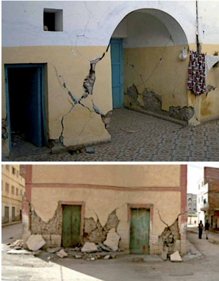
Figure 17. Examples of X-shaped damage clearly visible in a single-story class A house (above) and blurred by loss of outer leaf in a four-story residential block (below). Source: P Murphy.
