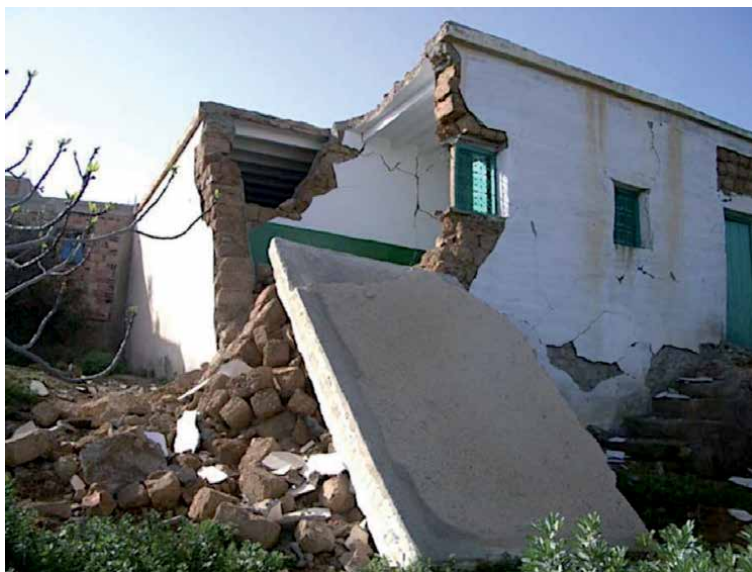
Figure 14. Ait Kamar, corner failure pulling down the roof slab (grade 4, class A). Source: P Murphy.
