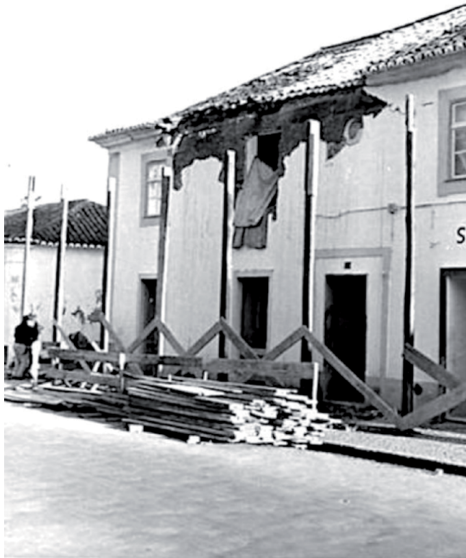
Figure 9. Portimão, two-story building of class B with detachment and toppling of the outer leaf of the external wall on the second floor, due to a hammering effect between the wooden joists supporting the roof and the top of the load-bearing walls (grade 3). The lack of shear cracks indicates a ground displacement from back to front. Source: IPMA.
