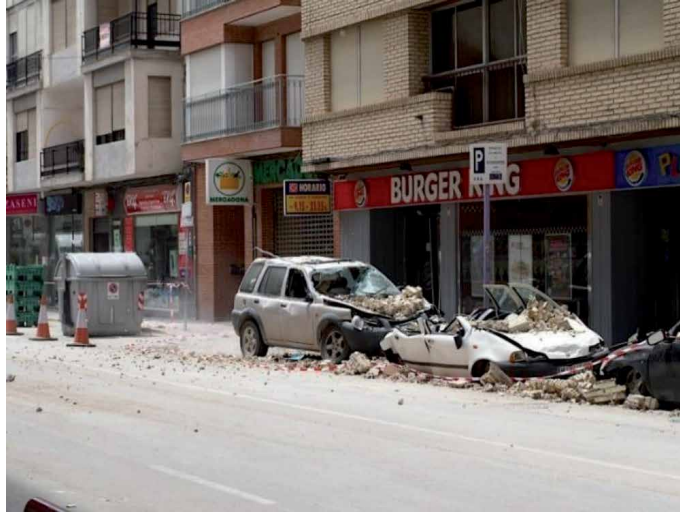
Figure 22. Lorca, debris fallen on vehicles and sidewalk. The center of the street is free of danger. In Lorca, people died while walking or looking for protection near the façades. Source: IERD.
