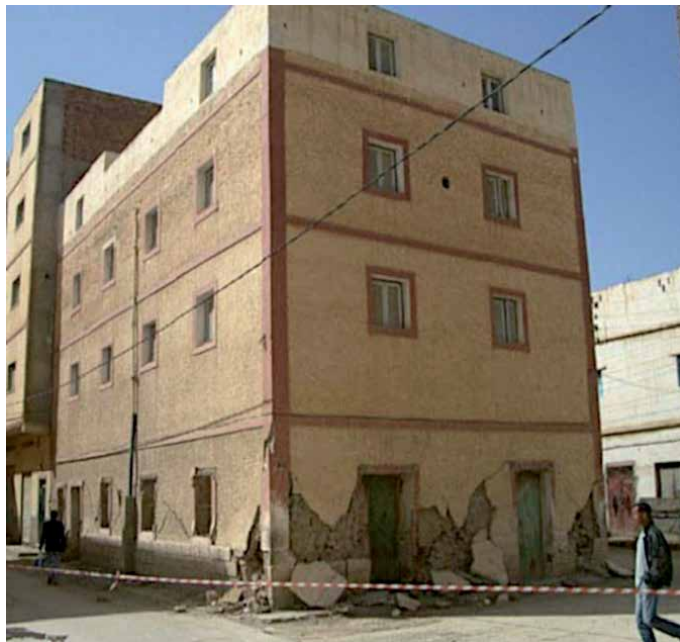
Figure 16. Imzourem, X-shaped damage completely surrounding the load-bearing walls on the ground floor of a four-story residential building of vulnerability class B (grade 3). Source: P Murphy.
