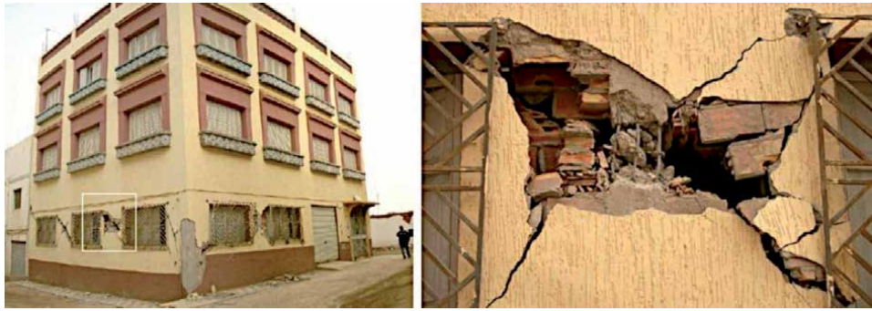
Figure 18. Imzourem, short column effect in a three-story residential block of vulnerability class C (grade 4). On the right, a detail of the damage is shown. Source: P Murphy.
