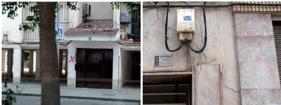
Figure 20. Lorca, shear cracks in pre-1968 RC buildings of class C (grade 3). There is apparently no evidence of structural damage, and on the ground floor (left) the columns forming an evident soft story have no sign of tilting. Source: IERD.
