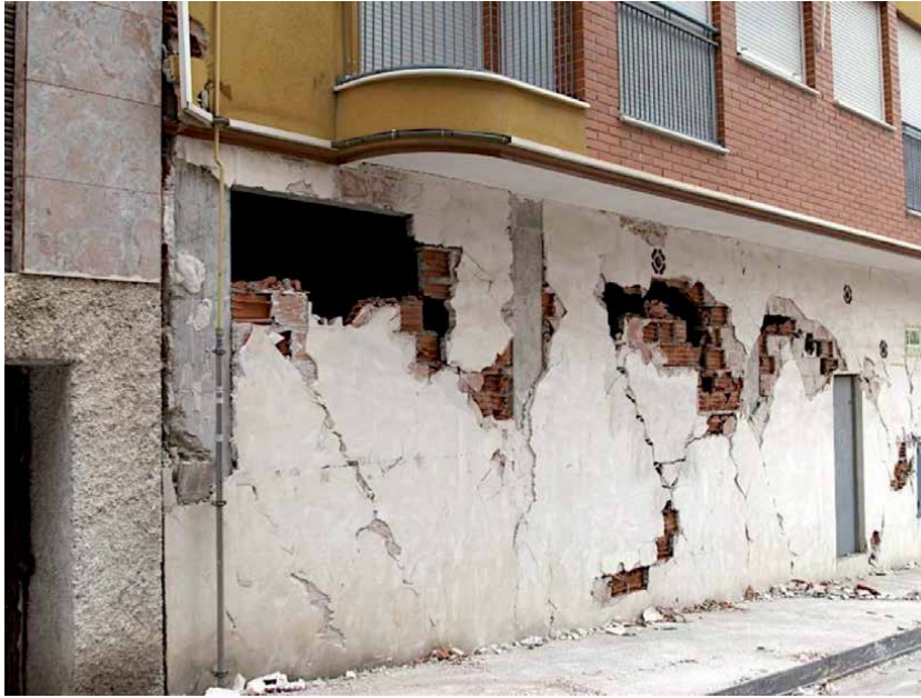
Figure 28. Lorca, X-shaped cracks in infill walls and loss of concrete in the middle body of the RC column suggest a soft story effect. Source: IERD.
