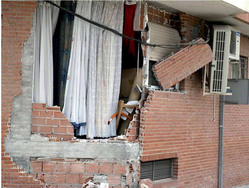
Figure 26. Lorca, complete overturning of double-leaf wall with overturning of both brickwork faces, but without apparent cracks in the RC frame. Source: IERD.
