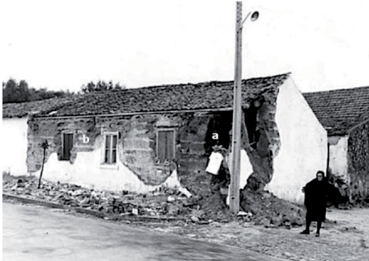
Figure 12. Grândola, damage of grade 4 in a house of class A (adobe masonry): (a) advanced corner failure not compromising the roof; (b) general detachment of plaster. Source: IPMA.
