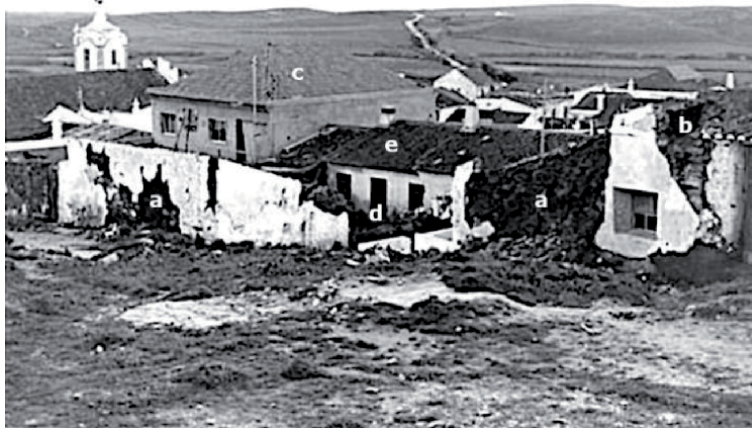
Figure 3. Vila do Bispo, general overview: (a) loss of the outer leaf of load-bearing walls and detachment of plaster; (b) partial toppling of façade wall, pulling down part of the roof; (c) good behavior of a recent construction (class B); (d) simple overturning of a freestanding masonry wall; (e) adobe house without apparent damage. Source: IPMA.
