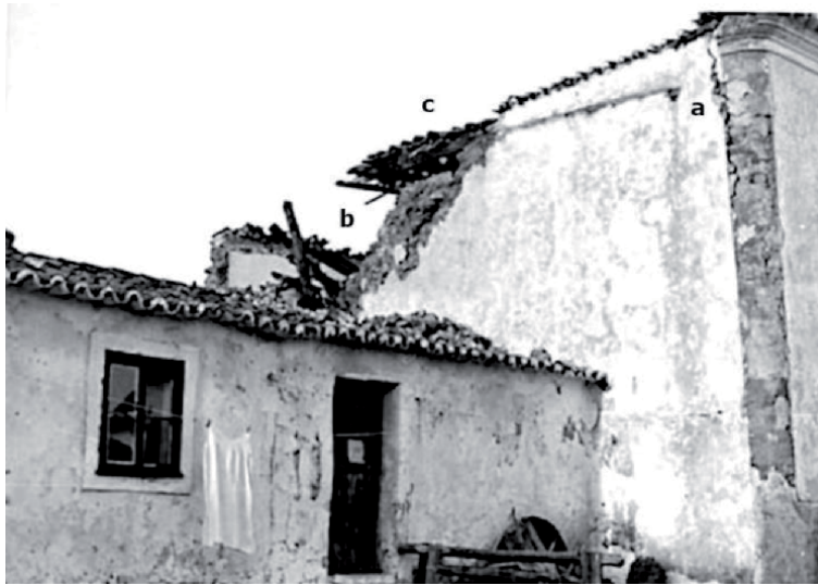
Figure 6. Vila do Bispo, building of class A with damage of grade 4: (a) loss of connection between load-bearing walls; (b) toppling of external wall; (c) collapse of roof made of wooden logs and bed of reeds. Source: IPMA.
