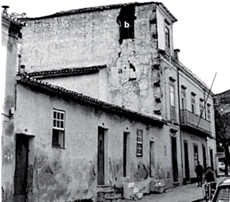
Figure 1. Silves, building of class B with damage of grade 3: (a) shear cracks with detachment of little pieces of plaster; (b) partial toppling of external wall. Source: IPMA.
