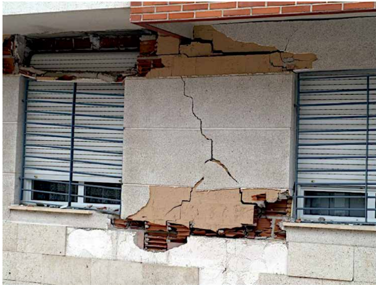
Figure 24. Lorca, loss of stone cladding, fall of window lintel and X-shaped crack on external wall about to fall down. Source: IERD.
