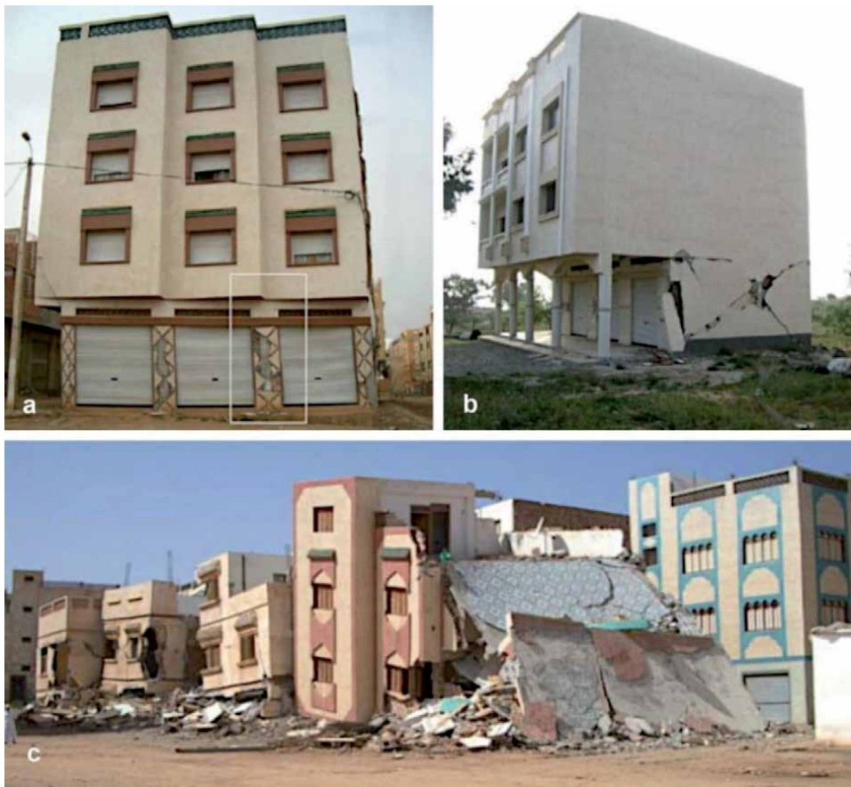
Figure 19. Alhucemas, soft-story failures: (a) tilting of RC frames on the ground floor; (b) soft-story damage with clear X-shaped crack on the infill wall; (c) collapse of ground floor due to a previous soft-story damage. Source: P Murphy.
