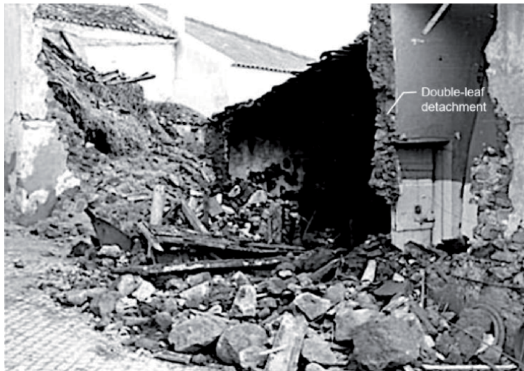
Figure 4. Vila do Bispo, total collapse of building of class A made of mixed fieldstone and adobe masonry, mud or clay mortar and roof supported by wooden logs and bed of reeds (grade 5). See the double-leaf shape on an interior load-bearing wall remaining standing. Source: IPMA.
