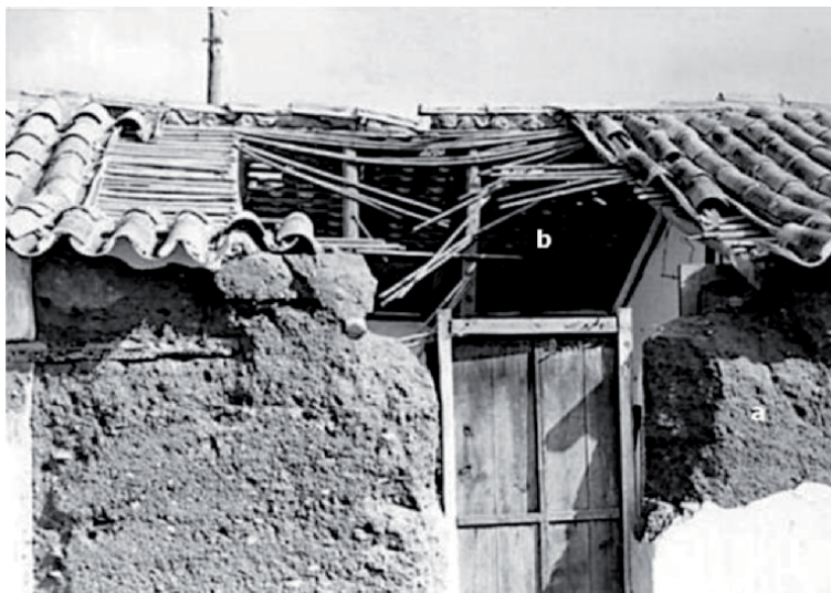
Figure 11. Odemira, damage of grade 4 in adobe masonry house of vulnerability class A: (a) detachment of plaster; (b) partial roof collapse due to the strong pounding of wooden logs against the top of the load-bearing wall. Source: IPMA.
