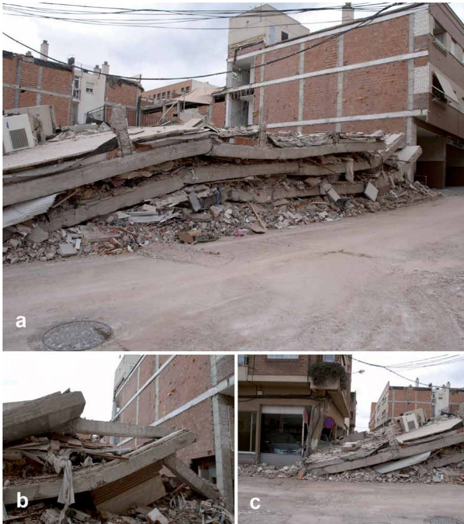
Figure 21. Lorca, complete collapse of RC residential building (grade 5) designed under the earthquake-resistant standard prior to the 2002 standard: (a) the three slabs are completely collapsed without any gap to allow survival; (b) plastic hinges and overturning in the direction of the slope of the street; and (c) plastic hinge in the adjacent building caused during the collapse, wedging against the base of the column. Source: IERD.
