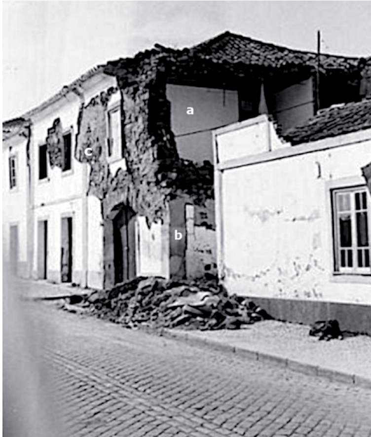
Figure 2. Bensafrim, building of class A with damage of grade 4: (a) advanced corner failure and toppling of external wall with partial roof collapse; (b) loss of connection and drift between load-bearing walls; (c) generalized detachment of plaster. Source: IPMA.
