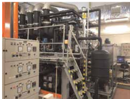
Figure 1. Adsorption cycle pilot installed at NUS, Singapore (published with PI permission [43, 44]).
