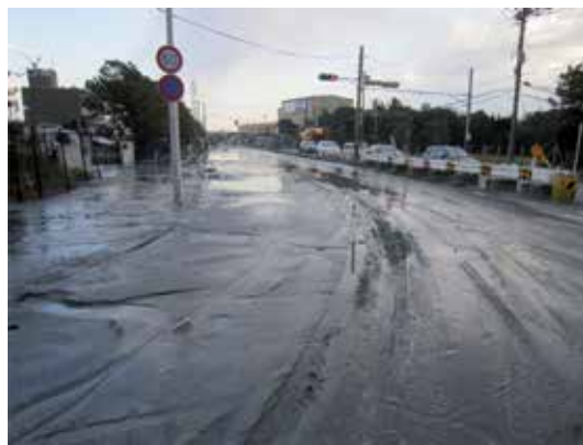
Figure 8. Liquefaction damage in Chiba Prefecture at East Japan (after Funabashi city data in Chiba Prefecture).
