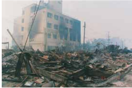
Figure 7. Collapses of buildings in Kobe at 1995 Kobe earthquake (after Kobe damage database).
