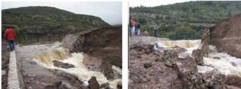
Figure 4. Overflow and failure of the spillway of the La Salitrera dam, in 2010.
