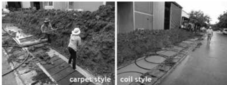
Figure 13. Installation of horizontal heat exchangers in Saraburi campus, Chulalongkorn University, Thailand (No. 7).
