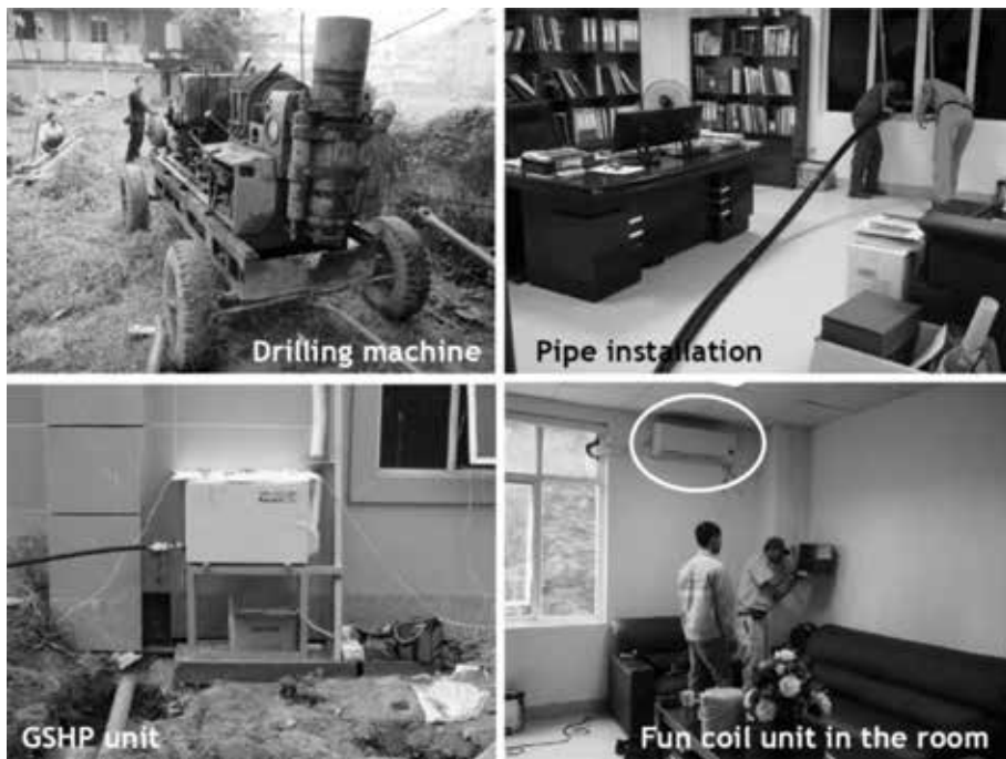
Figure 14. Installation of a GSHP system in Vietnam Institute of Geology and Mineral Resources (VIGMR), Hanoi, Vietnam (No. 9).
