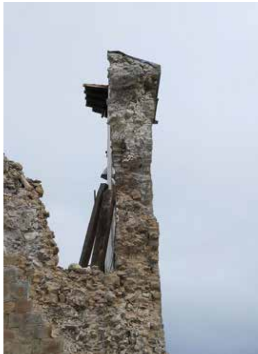
Figure 1. Collapse of the St. Agostino church in Amatrice after the Central Italy earthquake 2016 (image courtesy of the Curia of Rieti).
