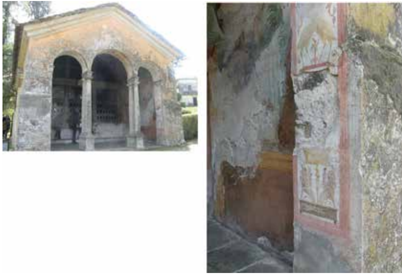
Figure 16. Decay of historical plasters because of the rain infiltrations (Sacro Monte of Varallo).
