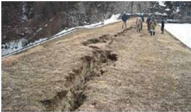
Figure 1. Crack at the Earth-fill dam.
