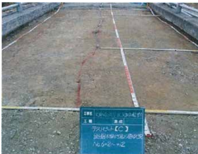
Figure 2. Crack at the rock-fill dam.
