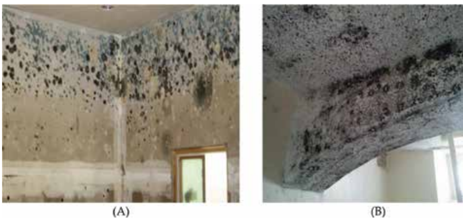
Plate 3. (A) Damped roof in a building in Bere Area of Ibadan, and (B) mould growth on wall and ceiling of a typical house in Ibadan.
