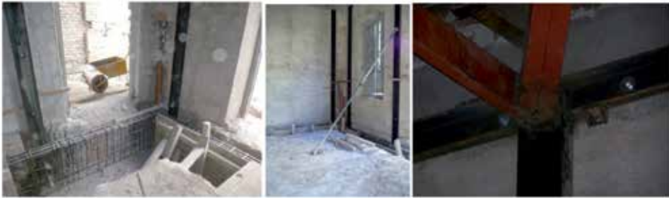
Figure 11. Reinforcement of foundations and reversible metallic structures in columns and lattice, Mitre school, 2012.
