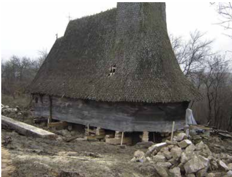
Figure 5. The lifting of the church.
