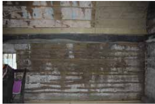
Figure 13. Degradation state of paintings near sampling point 10, 11, and 12.
