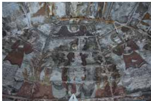
Figure 5. Semicap altar—degradation caused by humidity infiltration.
