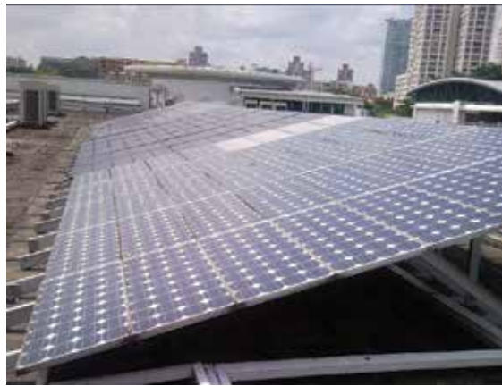
Figure 7. Conventional monocrystalline, polycrystalline and thin film (CIS) PV systems at CITI (BCA), Singapore [22].
