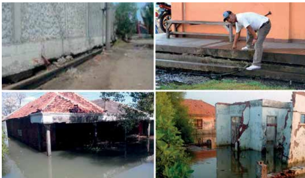
Figure 7. Pictures of the impact of subsidence (e.g. cracks in buildings and infrastructures and tidal inundation) in other regions of Indonesia (source: authors).
