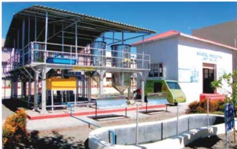
Figure 2. CO 2 capture & sequestration plant (CO 2 & steam source—oil fired baby boiler).
