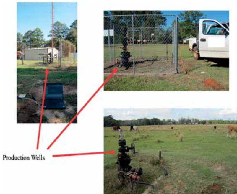
Figure 2. Typical locations of the oil wells at Citronelle, Alabama.
