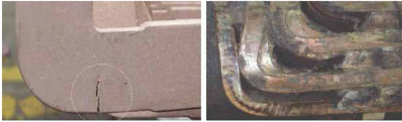
Figure 26. Cracking of copper turns and also bowing of the rotor.
