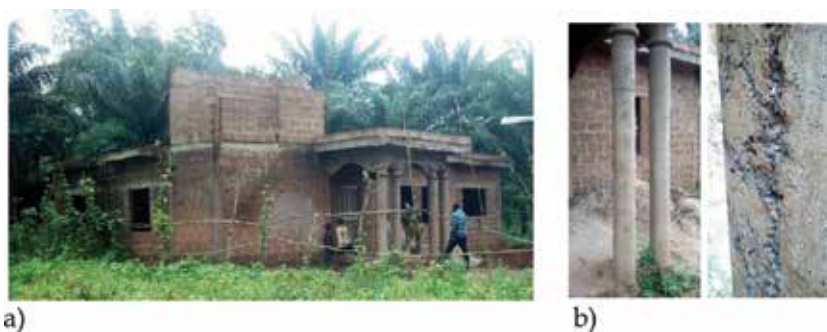
Figure 1. An example of a one-storeyed house in Missérété, constructed in 2014 with the use of OPKS concrete for the supporting elements. (a) Overview of the ongoing building. (b) Zoom on the columns of the main facade, showing on their surface the oil palm kernel shells in the cement matrix.
