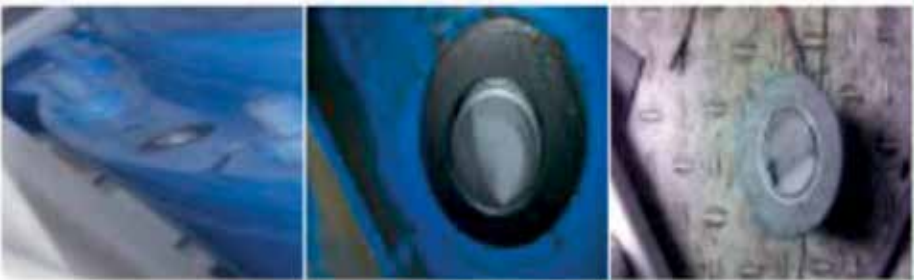
Figure 6. Bolt faults of wind turbine gearbox.
