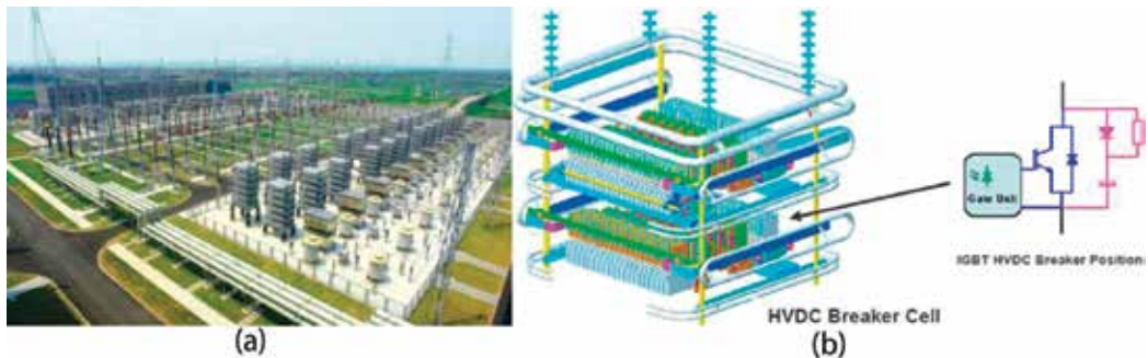
Figure 1. Two most important components in the flexible HVDC transmission system: (a) converter valve station and (b) schematic diagram for HVDC breaker [4].
