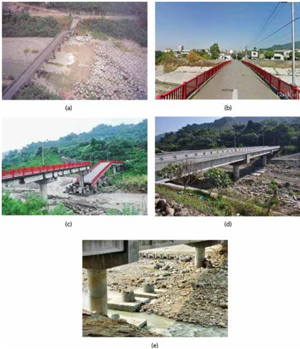
Figure 5. History of the Jianmin bridge in Taichung, Taiwan: (a) bridge collapsed during the Jiji earthquake, 1999 [10]; (b) bridge rebuilt in 2001 [11]; (c) bridge collapsed again in 2010; (d) bridge rebuilt again in 2012; (e) the exposed pile cap of the bridge [12].
