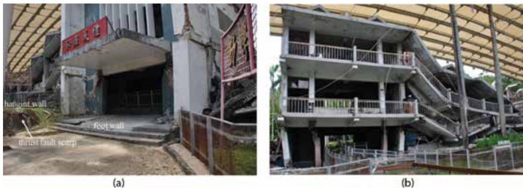
Figure 7. The collapse of the Kuangfu junior high school building during the Jiji earthquake: (a) front view; (b) rear view.
