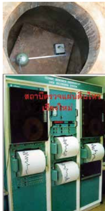
Figure 3. Installation of velocity sensor and accelerometer at CMMT seismic station (Thai Meteorological Department) [5].
