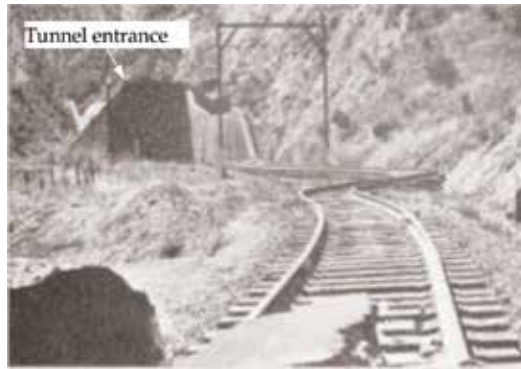
Figure 2. Damage at the tunnel entrance of the tunnel during the 1952 Kern country earthquake (adapted from [37]).
