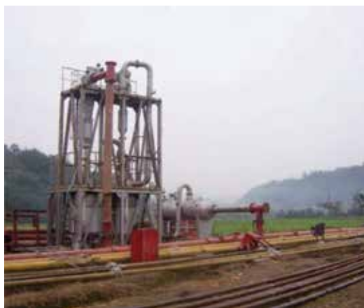
Figure 2. A gas recycling system installed in Sichuan province of China.
