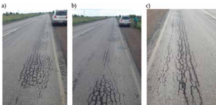
Figure 1. Fatigue failure of asphalt concrete pavement (860 km) of Karagandy-Shakhtinsk highway (Kazakhstan, Karagandy oblast, July, 2016).
