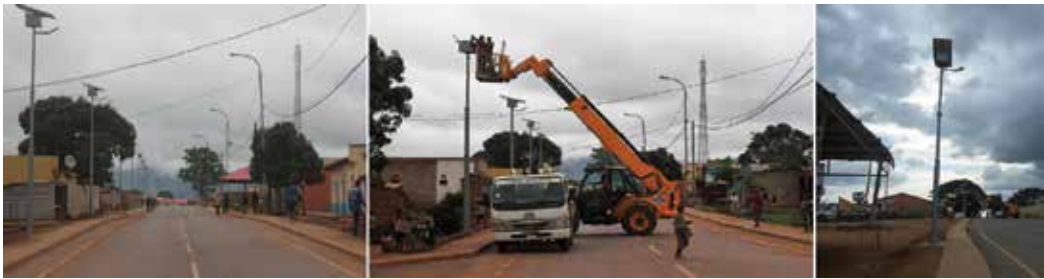
Figure 9. Solar autonomous public streetlight installation in Cuimba, Angola, 2017.
