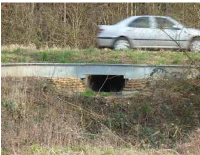
Figure 3. Ecopassage designed for the migration of amphibians along the road RD657 in NE France. This ecopassage allowed the migration of amphibians such as the common frog Rana temporaria and the common toad Bufo bufo . A concrete tunnel, with the floor covered by the soil, allows the animal crossing. A metallic barrier prevents the animals to access the road and directs them toward the tunnel entrance. This ecopassage is located below the local road joining Novéant-sur-Moselle to Arry in Northeastern France (photograph by Alain Morand, CEREMA-EST).
