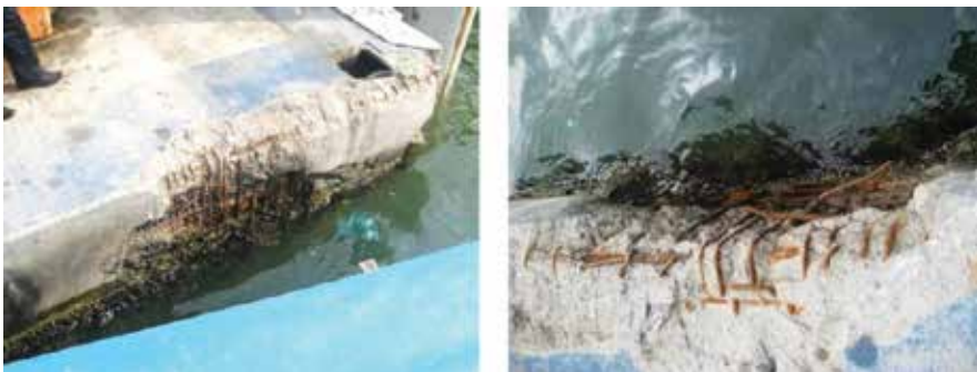
Figure 6. Corrosion of reinforced concrete in Qeshm port, Iran [45].
