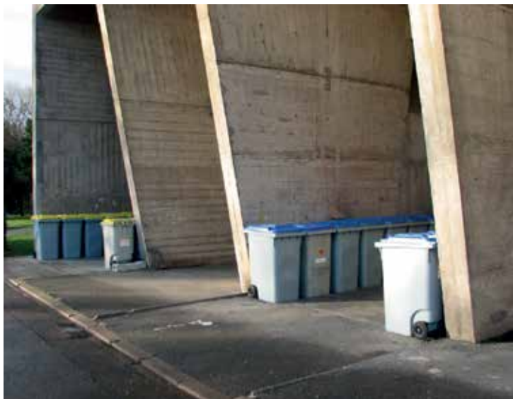
Figure 14. This is an image of the ground floor area le Corbusier structure in Rezé-Nantes and illustrates the realities of urban structures — Copyright © 2012, Jon Bryan Burley, all rights reserved, used by permission.
