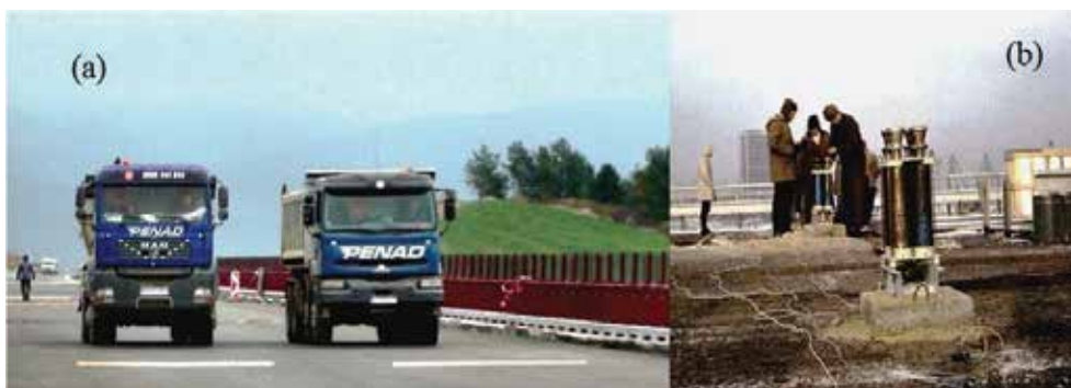
Figure 9. Testing load: (a) lorries traveling over the obstacles; (b) the PRE applied mainly on large bridge structure.
