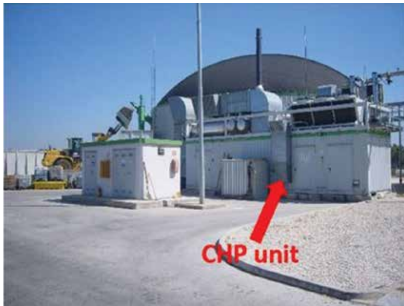
Figure 4. Combined heat and power unit (indoor place)—Source: Maccaresse S.p.a.
